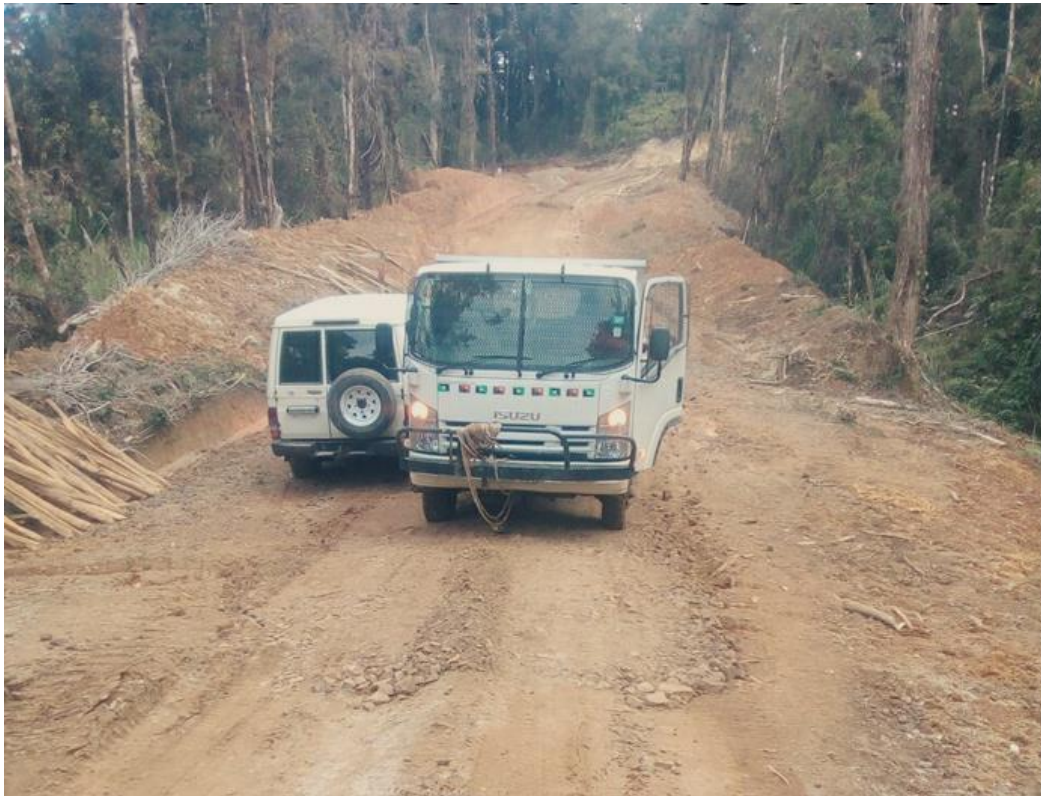
Figure 4: Crown Ridge all weather access road to camp, drill sites and sampling pits
