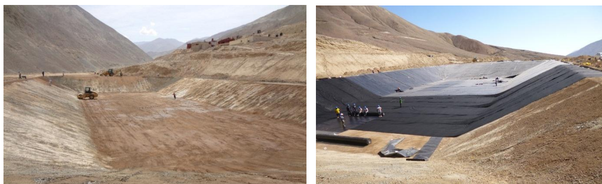
Figure 2: Construction of the initial tailings field, plant located in top right, and lining of the tailings dam (right).
