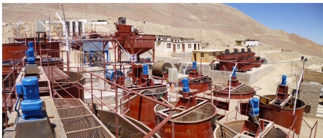
Figure 1: CIL and flotation circuits at the Mollehuaca Plant
